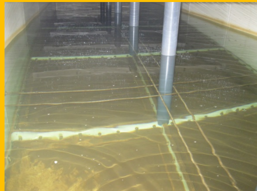
Slight surface scum indicating poor turnover and a significant level of debris. The tank should be cleaned and turnover monitored.
