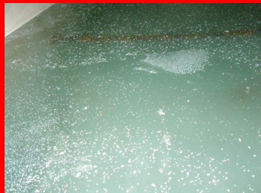
Severe stagnation indicating that the tank is unlikely to be required
