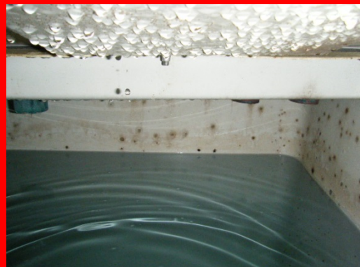
Gel coat failure resulting in local biological fouling (dark spots)
