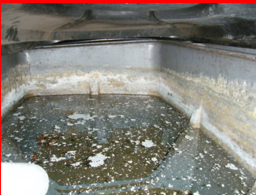
Unusually heavy scale formation requiring more than a regular clean and disinfection.
