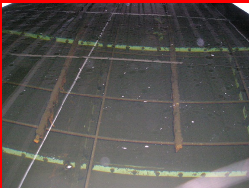
Heavy debris and corrosion internal parts that will require remedial works
