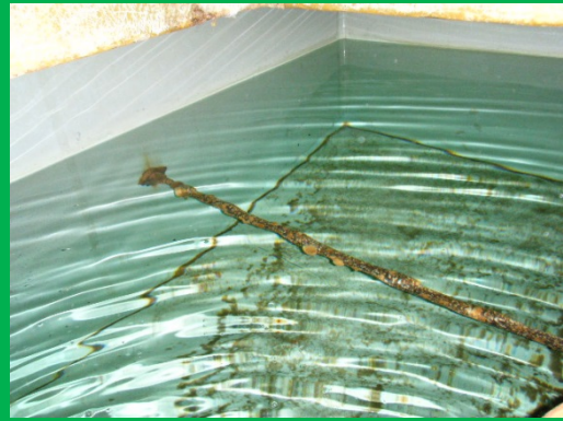
Light debris but corrosion to restraining bars
