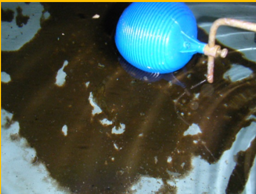
Moderate fouling suggesting cleaning should be conducted during the next 12 months
